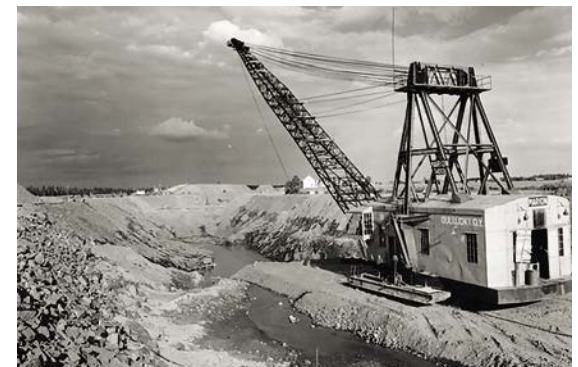
The largest crane working in Scandinavia. Photo: Fortum Oyj photo archive (U7 264 - 11.7.56)
