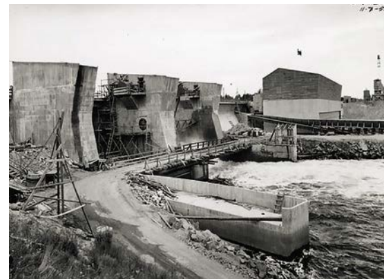
The dam on the left and power station on the right Photo: Fortum Oyj photo archive (U7 260 - 11.7.1956)
