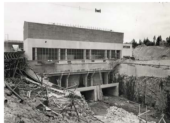
The power station and start of the tailrace. Photo: Fortum Oyj photo archive (U7 261 - 11.7.1956).
